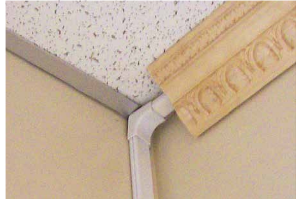
Ruggedized 3.0 mm Drop Cable shown behind molding
